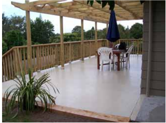
Category B structure: the deck hangs out from the house. No living structure underneath. Only the connection to the house is critical
